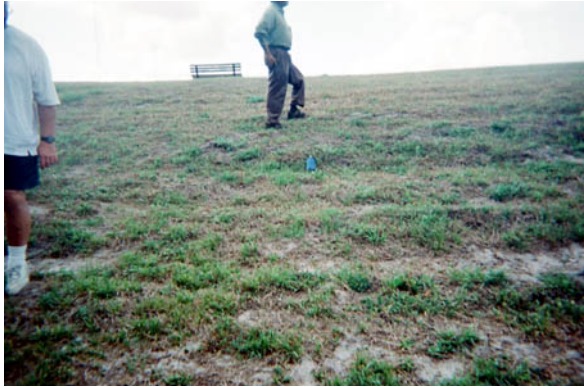
Ruts on north side of dam
