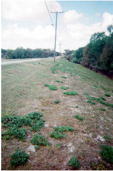
Ruts on north side of dam
