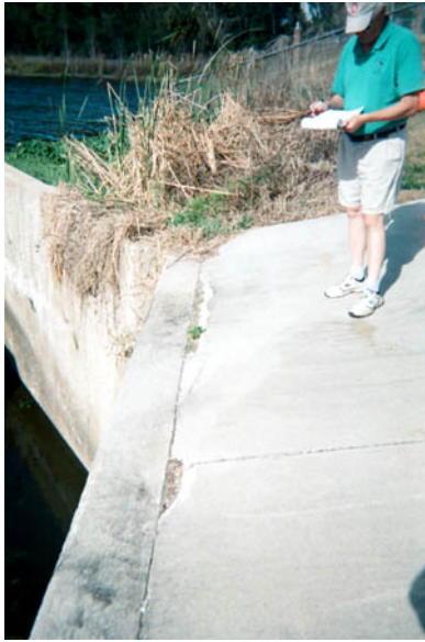
Cracked concrete seams
