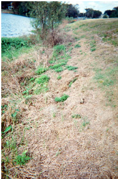
Ruts on south side of dam
