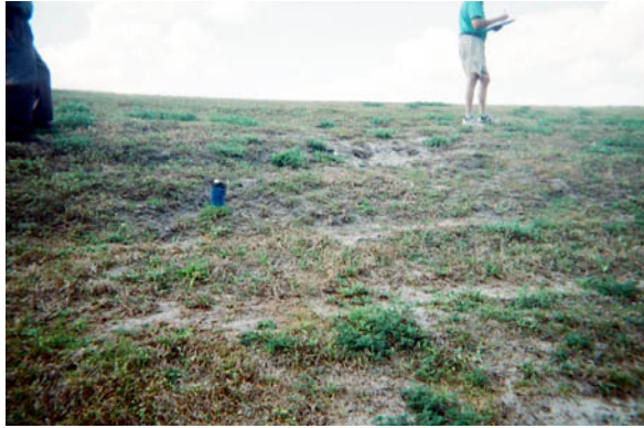
Ruts on north side of dam
