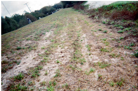
Ruts on south side of dam
