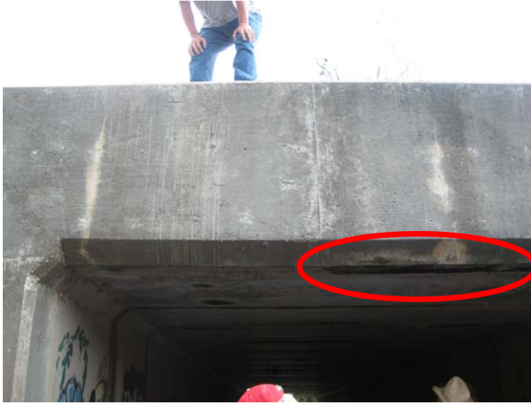
Item 6. Minor seepage.
