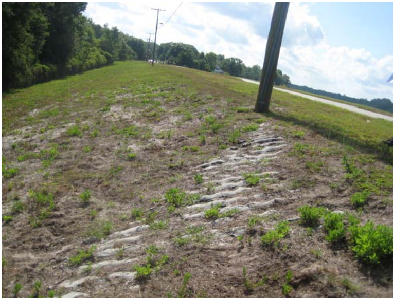
Item 8. Downslope erosion.
