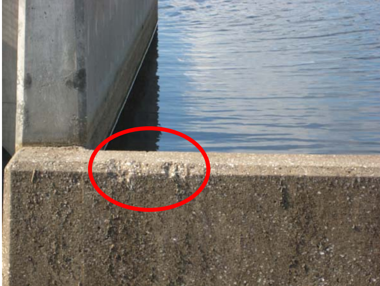
Item 5a. Concrete erosion/scarring.
